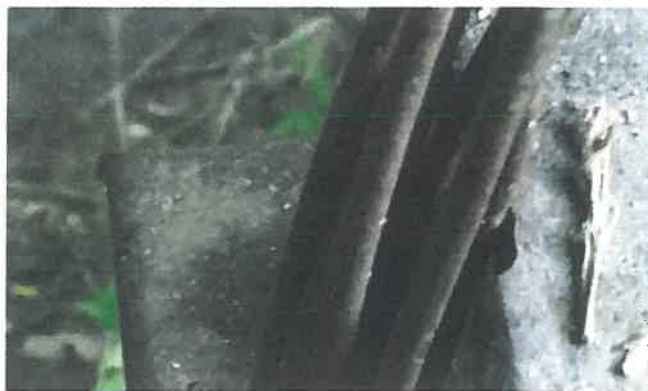
Note: gouge in top flange of floor beam 1 at hanger cable. This is one of the more extreme cases of gouging.
