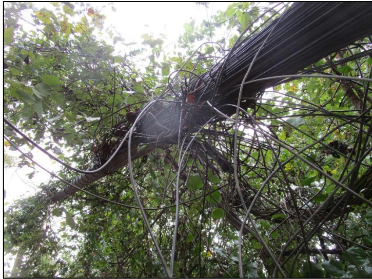
Southwest Main Cable Anchor-52 broken wires
