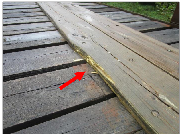
Runner Damage due to width
