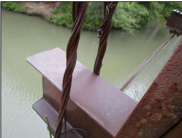
Hanger rubbing on Floorbeam Flange
