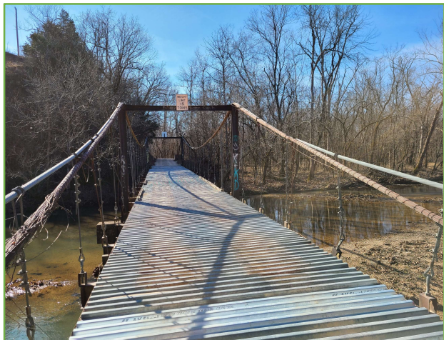
Figure 8 – Nearby Mill Creek bridge with 15 ton load limit was repaired in 1979 with new main cables, suspender cables, concrete anchorages and corrugated metal deck.
