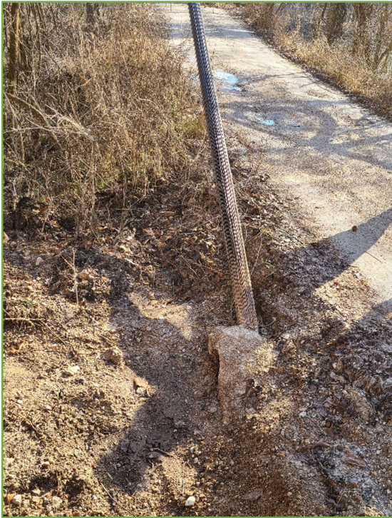
Figure 2 – Concrete anchorage at northwest corner of the bridge is being compromised by deterioration so new reinforced concrete anchorage must be constructed.
