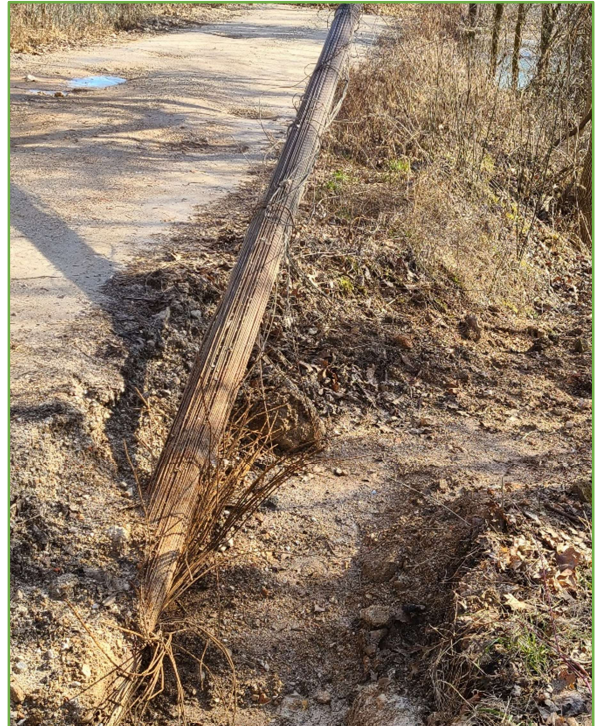
Figure 3 – Concrete anchorage at southwest corner of bridge is being compromised by deterioration so new reinforced concrete anchorage must be constructed.
