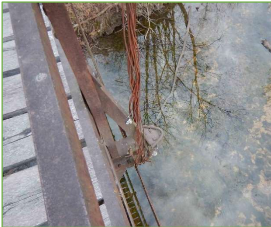
Figure 4 – Attachment details at top and bottom of replacement hanger cables can be improved. Rub-guard or saddle would slow the section loss in wires and floor beams. (MoDOT photo)
