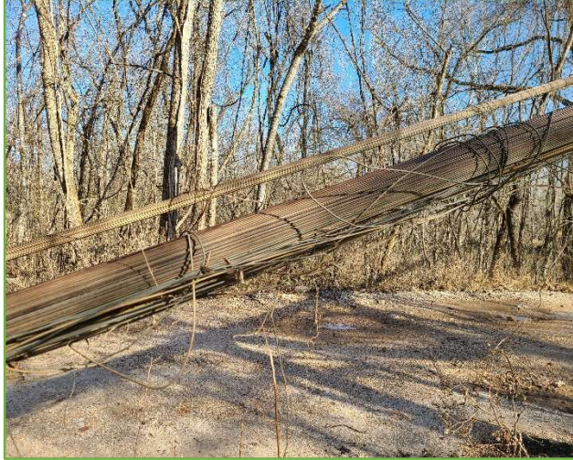
Figure 6 – Loose and broken outer wires are becoming more prevalent thus exposing the inner core and increasing the risk of being compromised.
