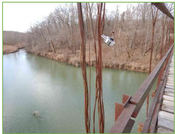
Figure 5 – Some hanger cables have become untwisted and lost tension; others have section loss or breakage in individual wires. (MoDOT photo)
