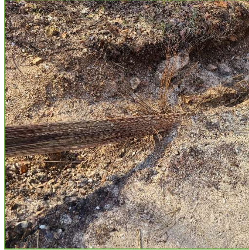
Figure 7 – Main cables at west anchorages no longer have outer wrap wires around a tightly bound core of individual wires.
